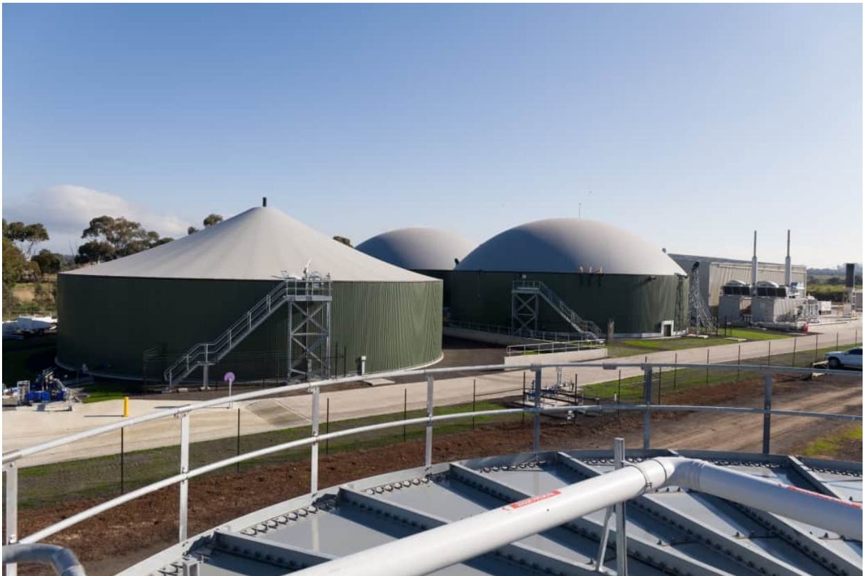
Figure 7: Digester tank at Wollert waste to energy facility
