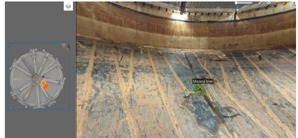
Figure 12 – Defect location and type on the internals of the tank
